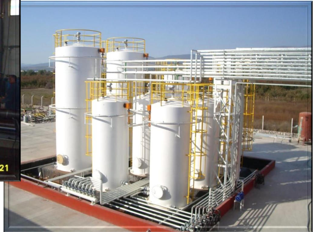
Solvent Storage Tanks
